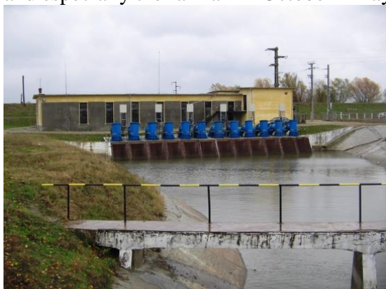
Figure 12 Cruceni pumping station (Photo: E.T. Man)
