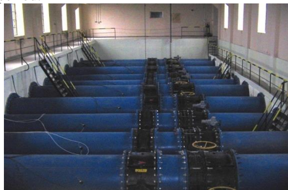
Figure 13 Pumps hall - Cruceni pumping station (Photo: E.T. Man)
